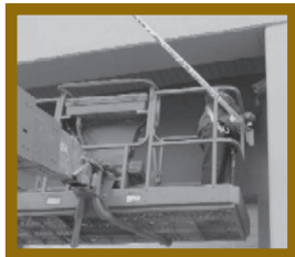
A 2005 incident involving an aerial platform lift indicates a common hazard while working under a roof (p. 23).
