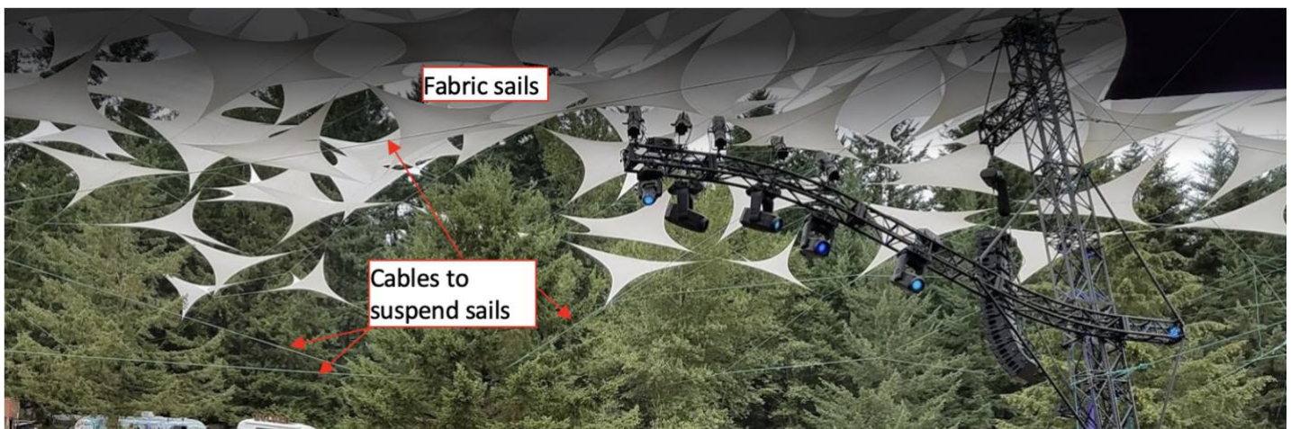
Image 1. Image of a fabric sails installation at the music festival venue. Note the cables attached to the sails are secured to trees in the background.
