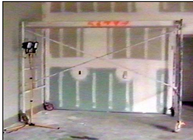
The scaffold used by the drywall installer and his lead man in this incident had only a single plank on the deck.
