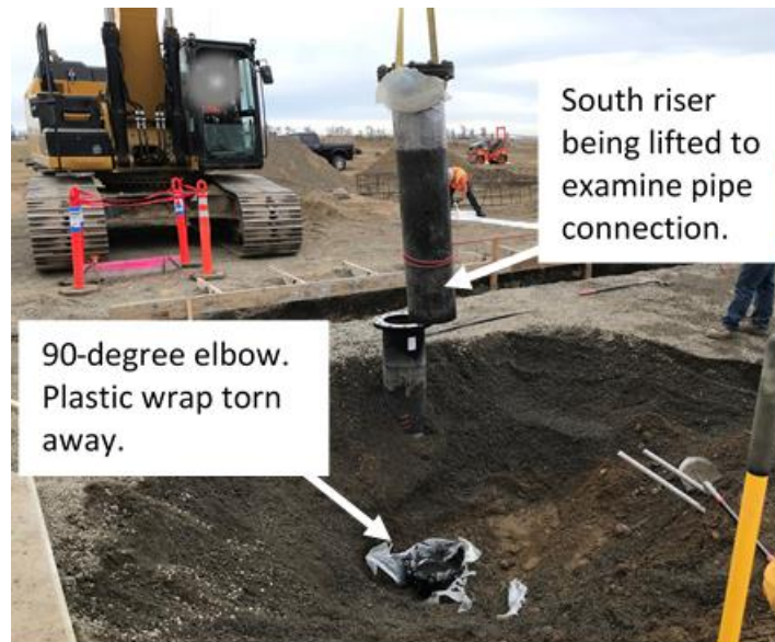
Photo 3. Post-incident excavation. South vertical riser to connection point with 90-degree elbow of horizontal pipe section. (Photo courtesy of OR-OSHA)
