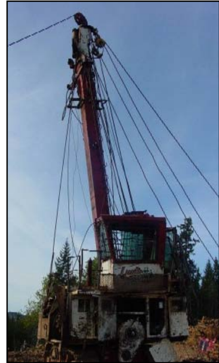
The yarder in this incident toppled over backward as the guylines were being spooled taut on the drums during setup.
