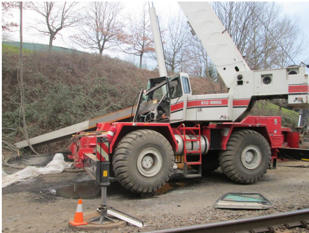
Figure1. Crane cab struck by H-beam.
