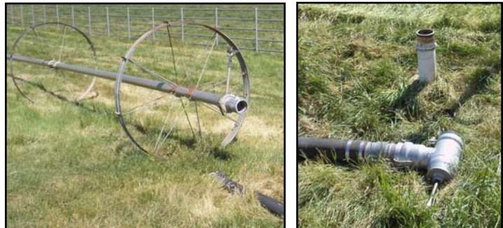
The irrigation wheel (left) connects to a heavy rubber supply line, which attaches to a removable valve (right foreground). The valve mounts over pressurized risers installed in the field, like the one shown here that failed (right background).
