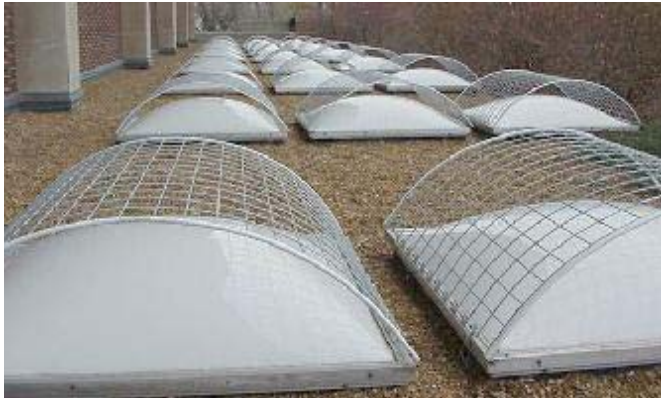
Photo. Skylight (typ.) with outer grids installed to prevent falls through them to the floor, below.
