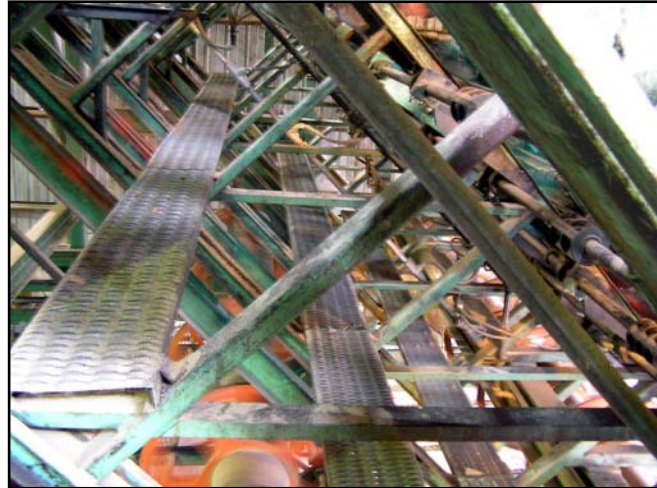
Catwalks in the tower planer provided access to areas where lumber occasionally jammed in the conveyor system.
