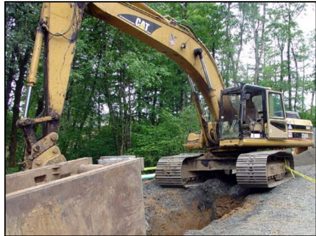
The track-hoe involved in this incident was pulling a trench shield forward in a trench for a sewer system when a hook failed and the rigging snapped loose.
