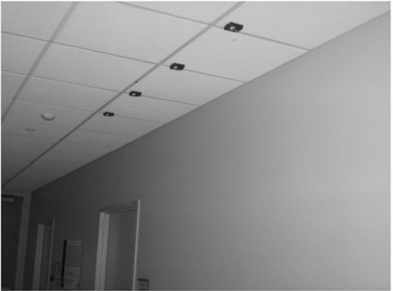
Fig. 1. A motion sensor line for measuring walking speed where the four sensors are placed 0.61 m apart and are installed on a ceiling typically 2.54 m high.
