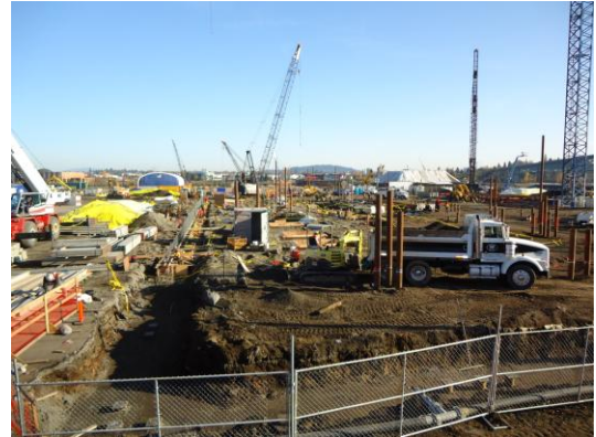
Here is how the under-construction OUS/OHSU Collaborative Life Sciences Building looked as of mid-December. The North tower, which will house the dental school come fall of 2014, is on the left. (Photo Sydney Clevenauer)
